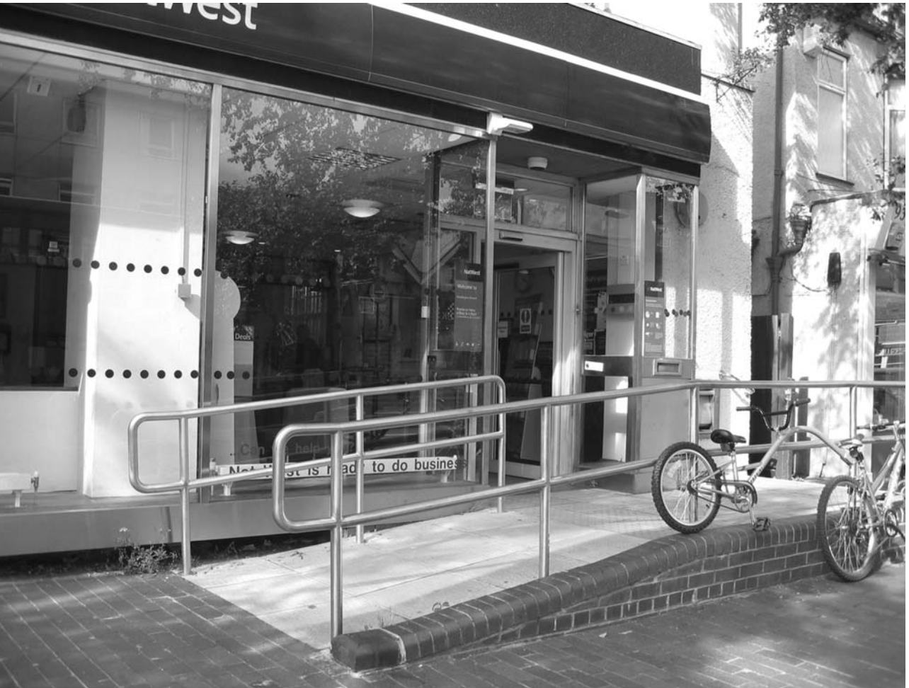
Figure 7.7 Ideally, even small changes in level should have both a ramp and steps.
