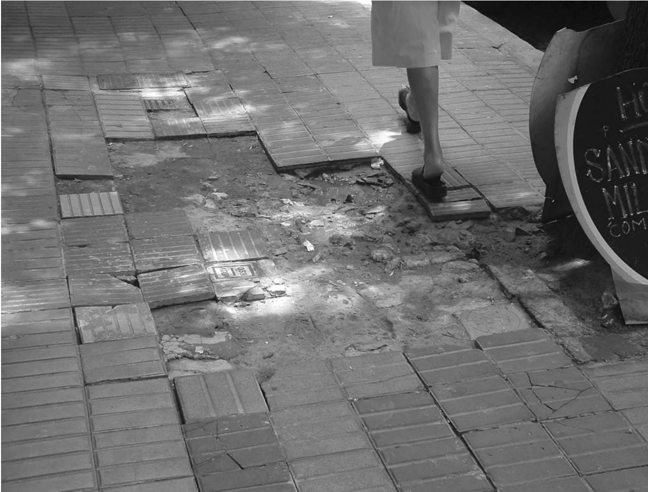
Figure 9.2 Older people find broken or uneven parking particularly hazardous.
